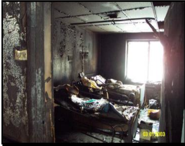
Figure 5 - Patient room (204) where the door was open during the fire (NFPA)
