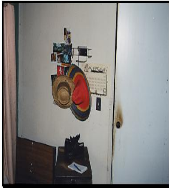
Figure 7 - Interior of patient room, where the door was closed during the fire (NFPA)
